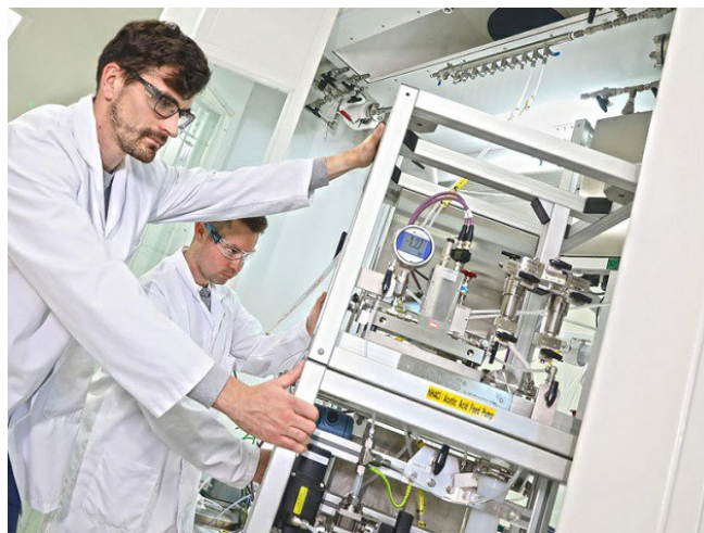
Liquid Dosing skid with CORI-FLOW (copyright: ISPE)
